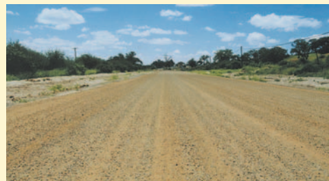
Otta Seal surfacing, 2 - 3 days after construction, and where traffic has been allowed using the surfacing immediately after construction. (Botswana).
