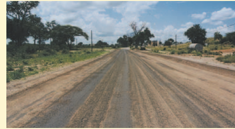
Aggregate that has been dislodged by traffic should be broomed back into the wheel paths. This to ensure maximum embedment of the aggregate into the soft binder. (Botswana).
