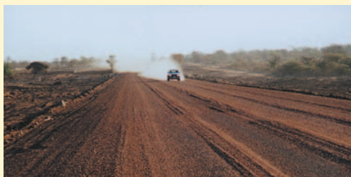
A too excessive aggregate application. (Botswana).
