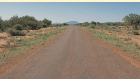
Overview of the same road (Single Otta Seal) after being in service for more than 8 years. (Botswana).
