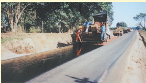
Otta Seals trial, using crushed quartzite with a high amount of fines. The aggregate was applied by a self-propelled chip spreader. (South Africa).
