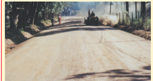
Preparatory work prior to sealing operation, cleaning loose material from the base. (South Africa).
