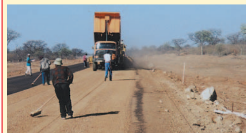
Otta sealing operations. Enough aggregate is essential in order to allow the binder to work its way upwards to coat all the particles. (Botswana).
