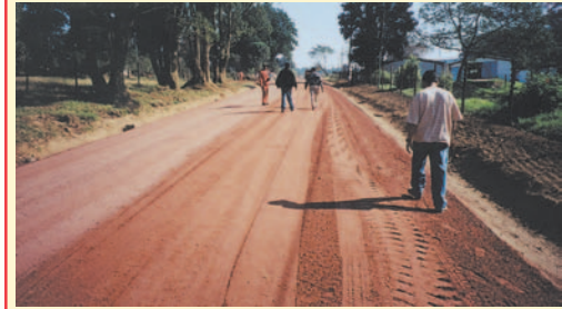
Immediately after the Otta Seal aggregate has been applied. The seal looks like a gravel road at this stage. But with time, the single Otta Seal will "bed down" and a bit premix type appearance will appear. (South Africa).
