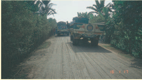
In the absence of pneumatic tired rollers, rolling of the Otta Seal can be done by loaded trucks following a pre-determined pattern of rolling. (Bangladesh).
