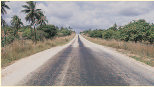
A section where coral stone was used as Otta Seal aggregate. The first section has been in service for some months and the aggregate has "bed down" making an appealing and uniform appearance. The second section has newly been constructed and the coral aggregate still need some time to "bed down". After more than 14 years in service these sections are performing excellently. (Kenya).
